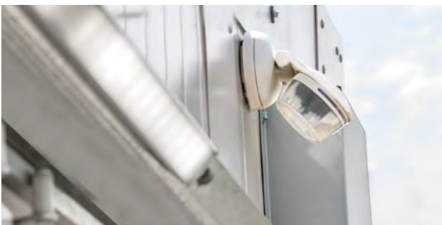
External lighting with motion sensor
