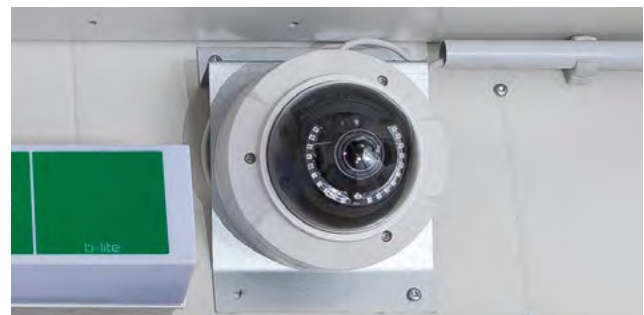
Video surveillance and recording of the hazard area indoors or outdoors
